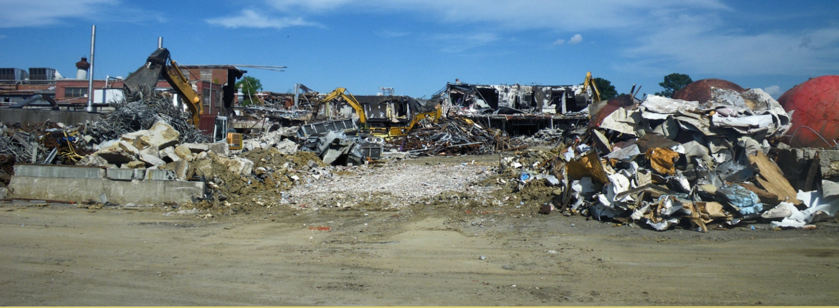
Multiple four story buildings demolished, along with six story water towers.
