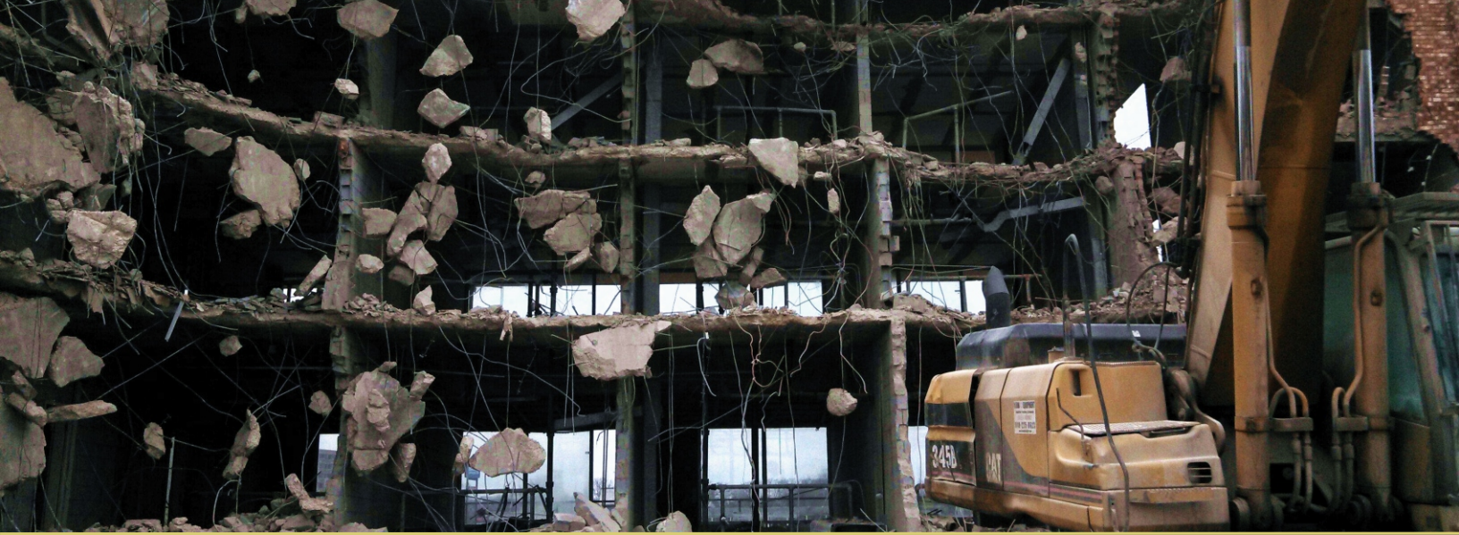
Environmental Abatement, Structural Demolition, Site Work: From an eyesore to Green Space
